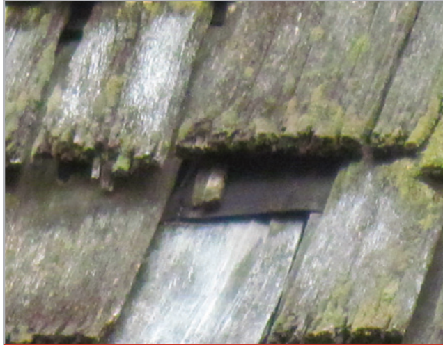
MISSING OR LOOSE SHAKES?
